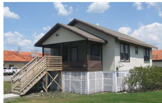
Soil below the stairway was lost as a result of subsidence.
