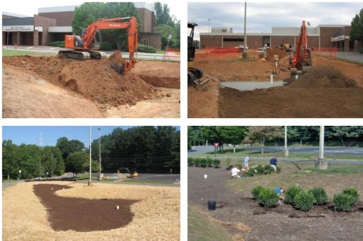
FIGURE 3. BIOFILTER CONSTRUCTION SEQUENCE. TOP LEFT: EXCAVATION OF BOWL CONTOURS; TOP RIGHT: FILLING BOWL WITH GRAVEL LAYER AND BIOFILTER MEDIA; BOTTOM LEFT: SITE STABILIZATION; BOTTOM RIGHT: PLANTING WITH FACILITATIVE WET PLANTS
