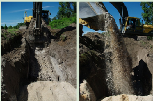
Excavation of denitrification wall trench (left) and backfilling with 50:50 sand:sawdust media (right)
