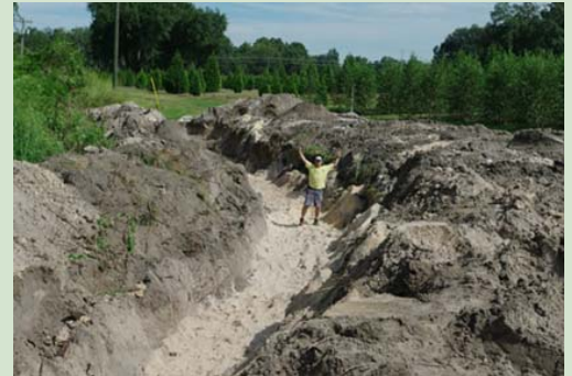
Denitrification wall trench excavation and backfill with sand:sawdust media completed. Topsoil was later backfilled on top of the denitrification wall media.
