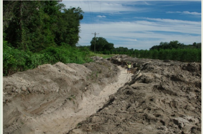
Denitrification wall with Casey Schmidt standing on 1.7 meters of sand sawdust mix prior to backfill
