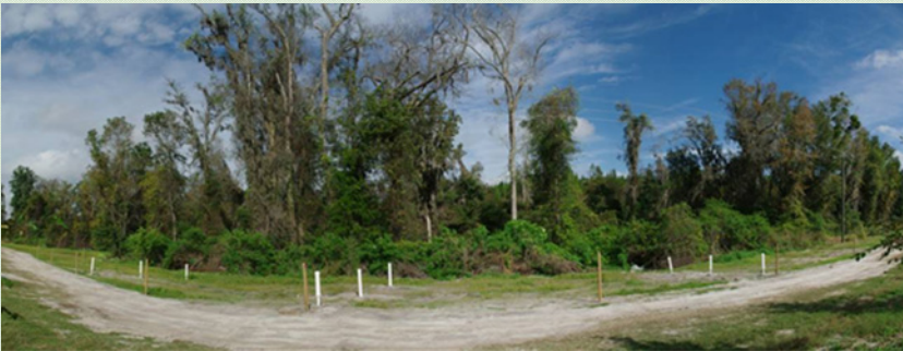
Finished denitrification wall looking downstream with three monitoring well transects identified by white PVC pipe. Monitoring transects are perpendicular to the wall with the middle well of each transect demarcating the center of the wall. Bare soil in foreground is a road
