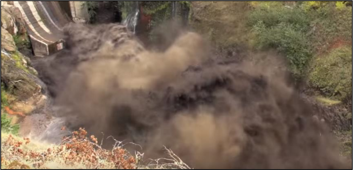
Figure 25: The release of the Condit Dam, massive black sediment filled water mixed with smoke from exploding dynamite and concrete create a black cloud.
