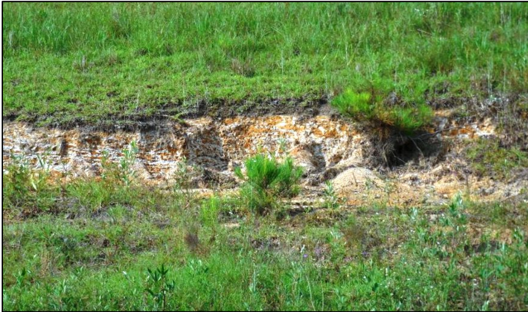
Fig. 1-1. I-10 right-of-way on embankment. Bahiagrass decline, followed by erosion and weed infestation exposes increasingly more soil over time.
