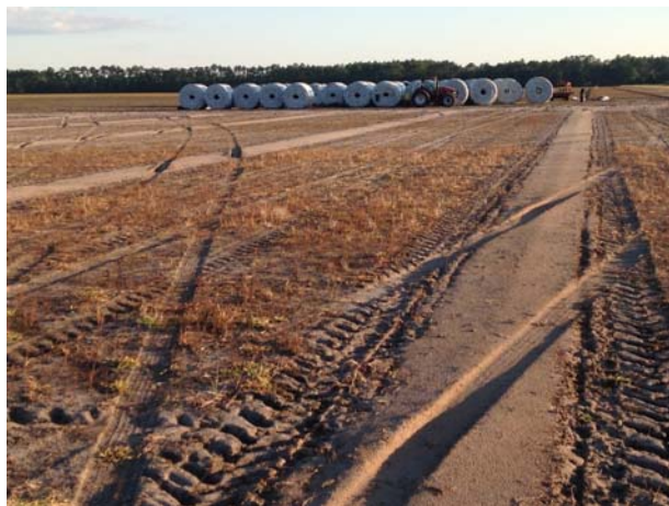
Installation of alternative irrigation and drainage system ("irridrain"). Seen are rolls of irridrain pipe (background) and the filled trench where it was installed (foreground).
