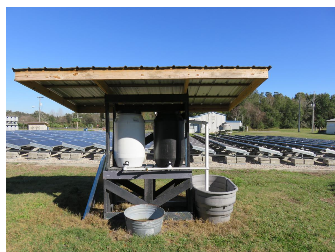
Stand-alone rainwater harvester at UF Bioenergy and Sustainable Technology Lab
