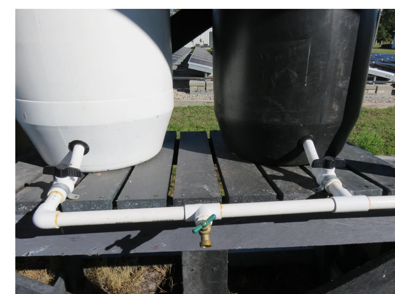
100-gallon storage capacity integrated within the infrastructure of the RWH
